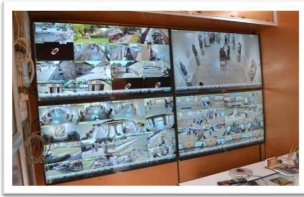
Monitoring unit of Installed CCTV Cameras
